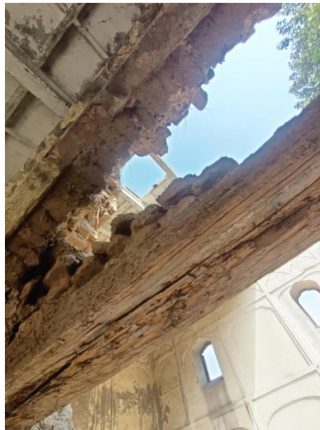
Figure 1 I: Broken roof of the Main Entrance Hall
