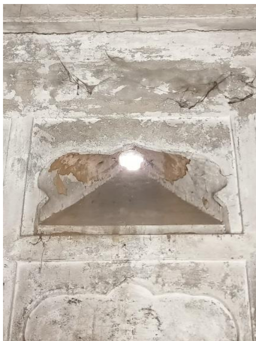
Figure 15: Open vents should be closed to avoid further damage
