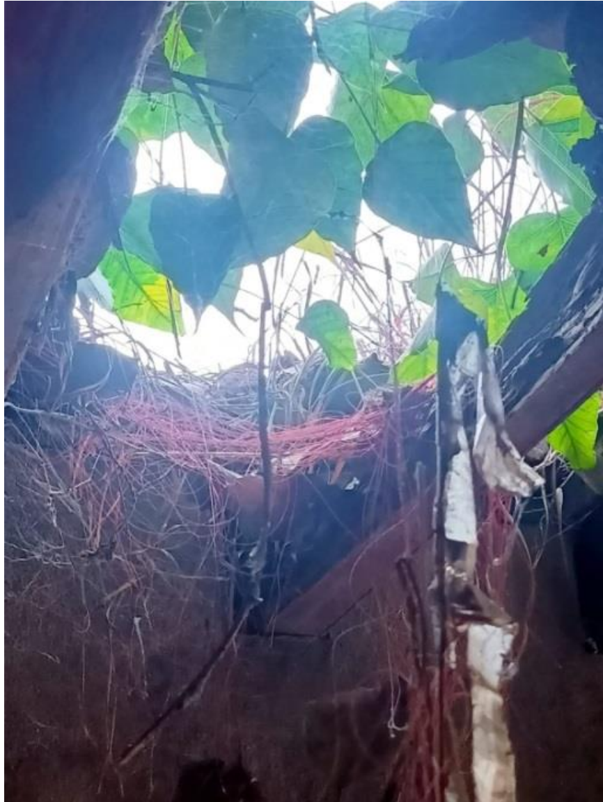
Figure 14: Leaves hanging from the holes on the roof of the staircase
