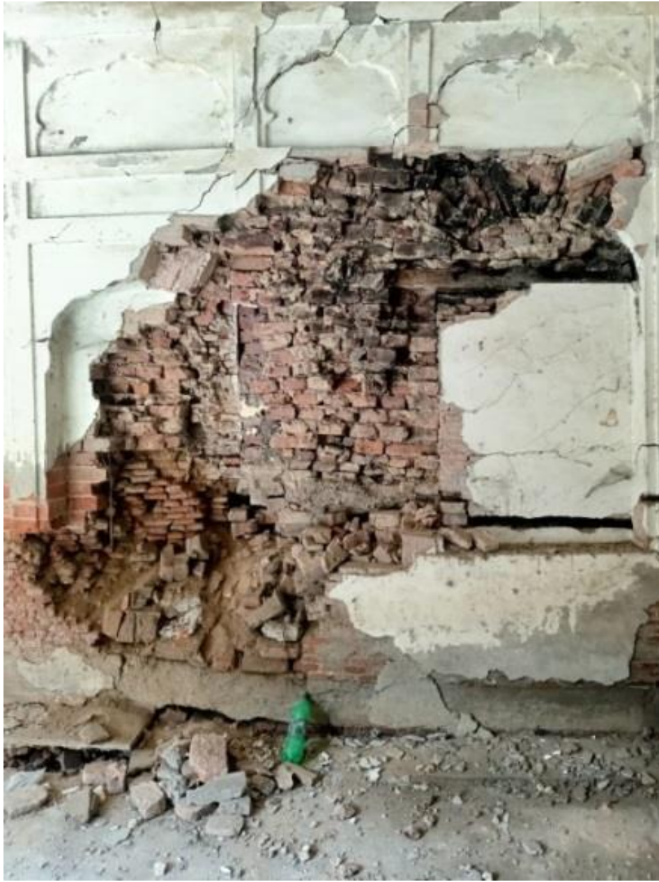
Figure 13: Broken walls and floor of the rooms
