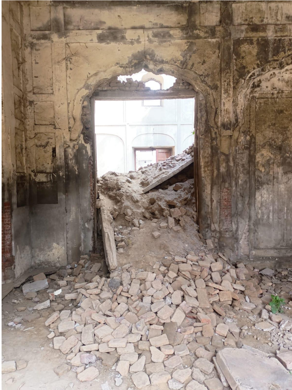
Figure I2: Need to clean extra and broken material
